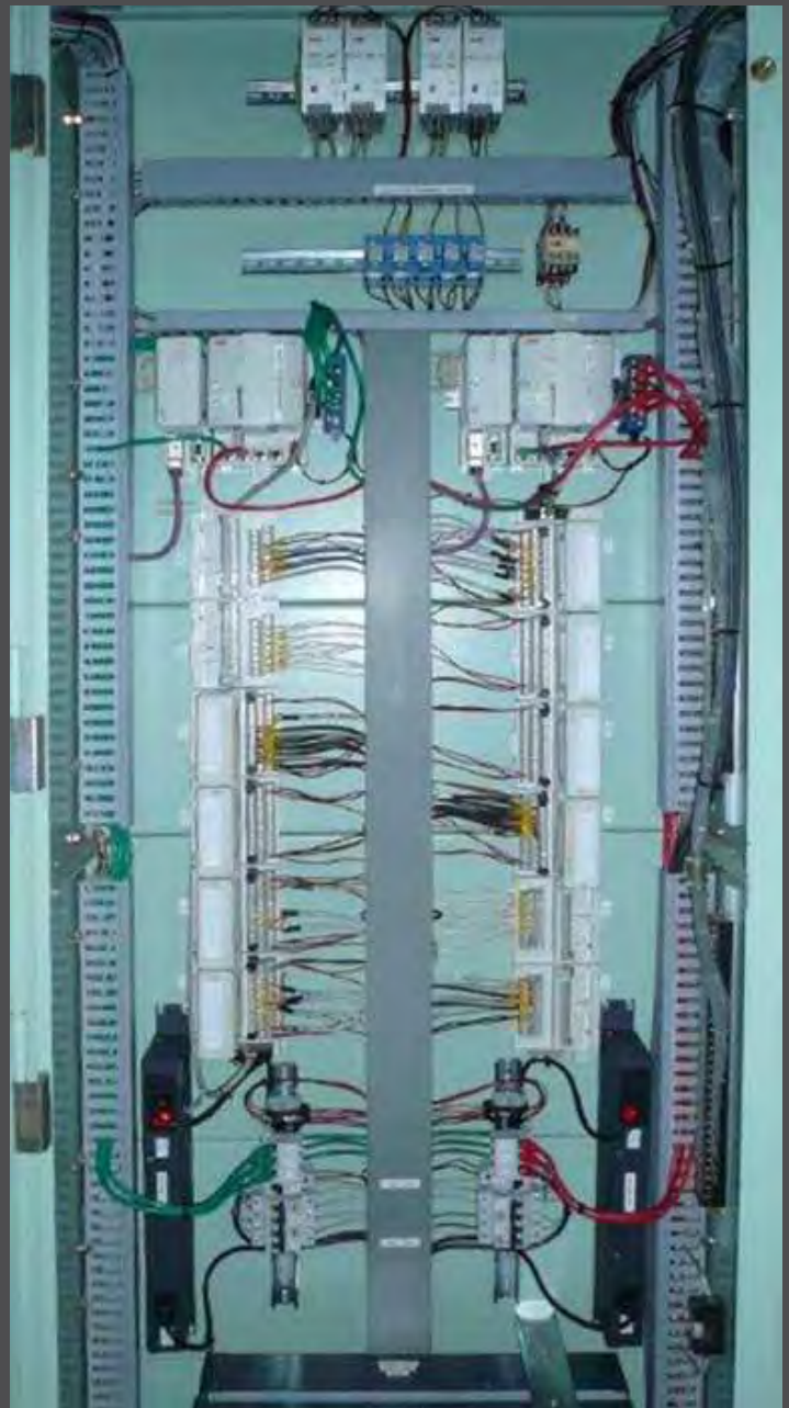
PFC-200 Node/ IO in a 3KV MSB
